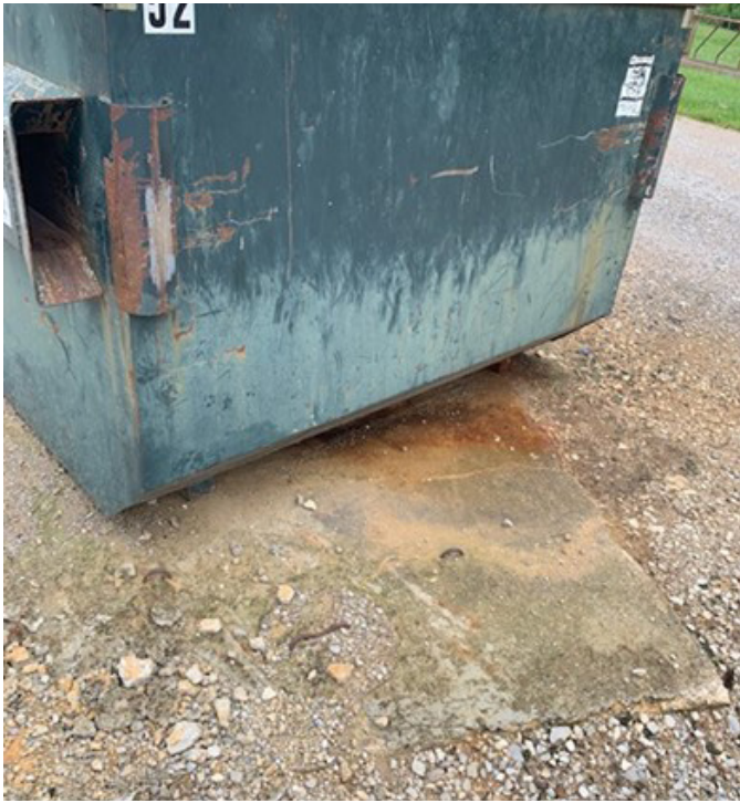
Dumpster covering broken septic tank
