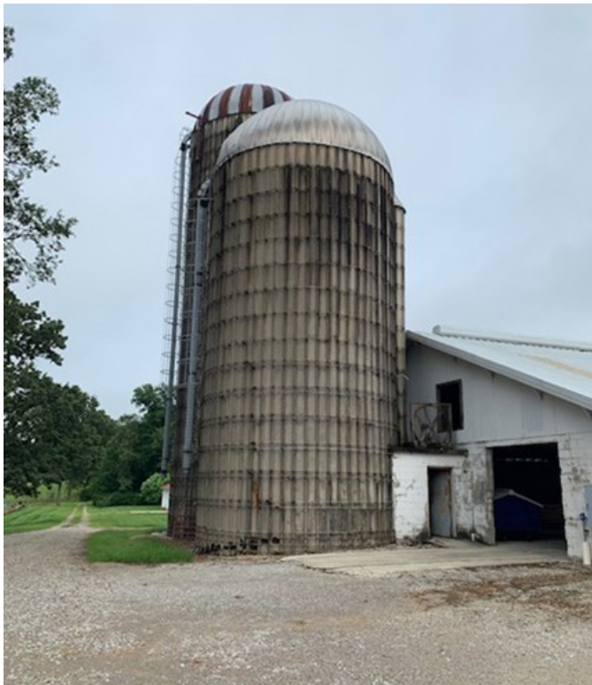
Structurally insecure silos See all the holes at the bottom?
